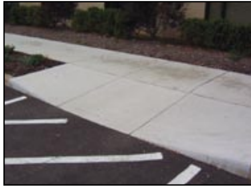
The proper design of this curb ramp in Warren meets all necessary requirements. (Photos by Marilyn Sydow)
