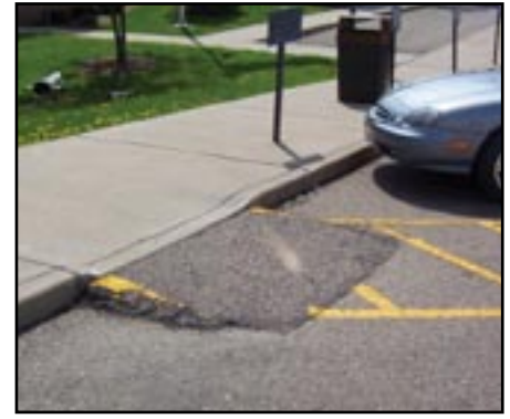
Built-up curb ramps (whether poorly-done or well-designed) should not be placed in handicap parking access aisles.
