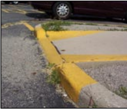
Instead of being flush, this curb ramp has a lip where it meets the asphalt, making the transition from parking lot to ramp abrupt.
