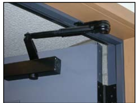
One of several door closer configurations, this photo depicts a surface mounted door closer with a double lever parallel arm connected to the top of the door frame.
